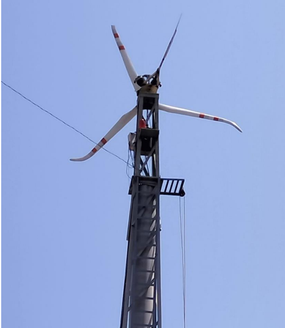
Fig 4: Platform and Pulley for maintenance
