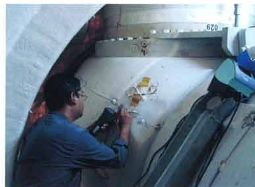
Rotor Instrumentation work carried out for WinWinD Power Energy for 1 MW Wind Turbine at Vengal, Chennai
