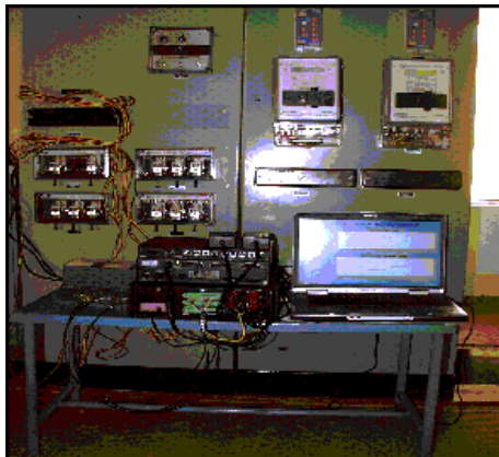
Measurement set-up at sub-station
