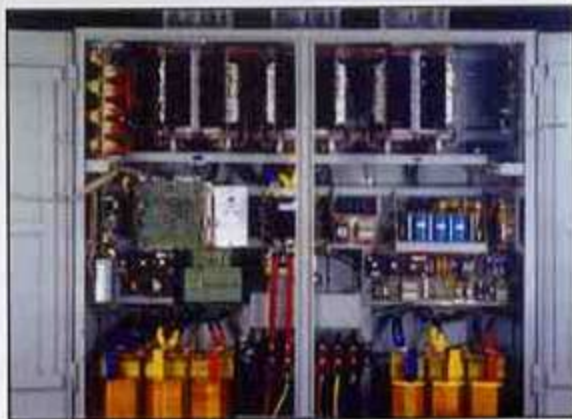
Intelligent Wind Controller designed and developed indigenously, installed in Wind Turbine at Muppandal, Tamil Nadu.
