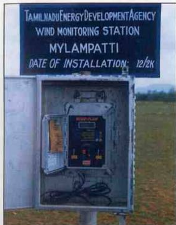
Close-up view of the NRG data logger installed at Mylampatti, Tamil Nadu
