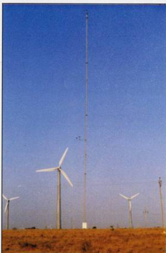
The 25m reference Wind Monitoring Station at Kayathar
