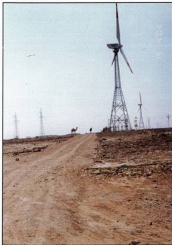
1000 kW Wind Turbine near Jaisalmer
