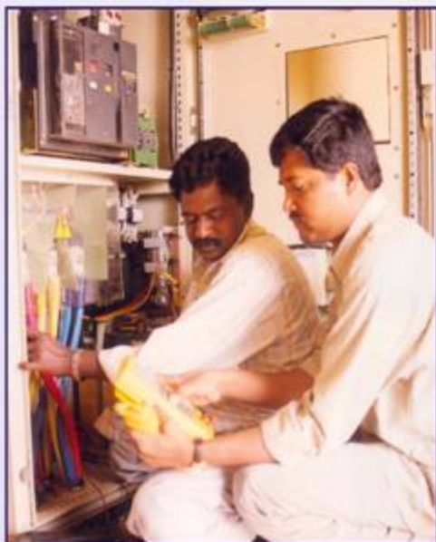
Verification of instrumentation on Suzlon 1000 kW wind turbine at Jaisalmer.
