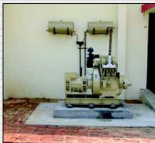
Fig.10: 20 kW Pungam oil generator
