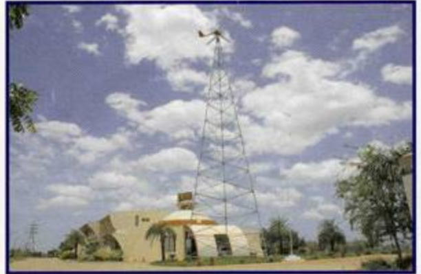
5 kW Wind Battery Charger installed in C-WET Campus
