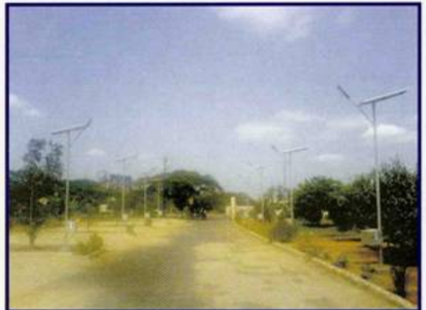
Solar street lights installed in C-WET campus
