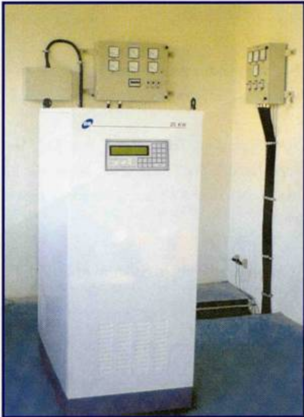
Power Conditioning Unit
