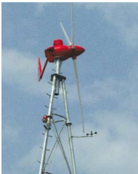
5 kW Battery charger Wind-Solar-Pungham oil Trigeneration System.
