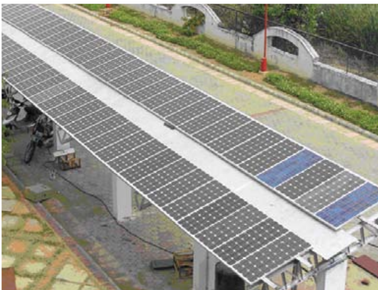
Solar Photovoltaic Panels
