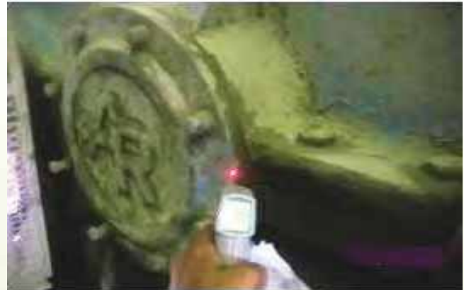
Temperature Measurement underway
