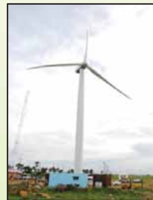
2 MW Kenersys make R&D Wind Turbine
