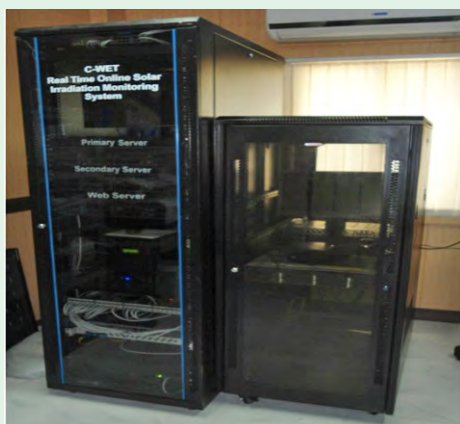
Level-1 & Level-2 Servers at CRS
