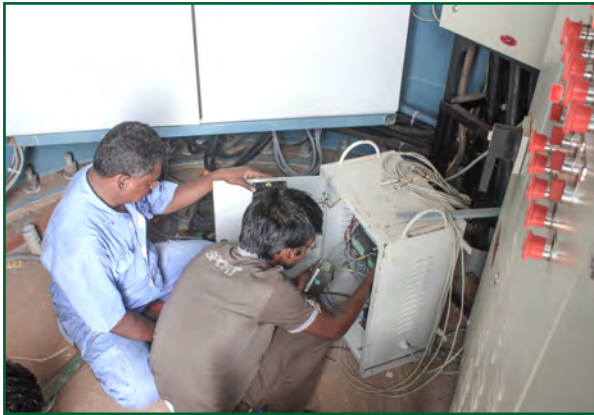
Power Transducer wiring
