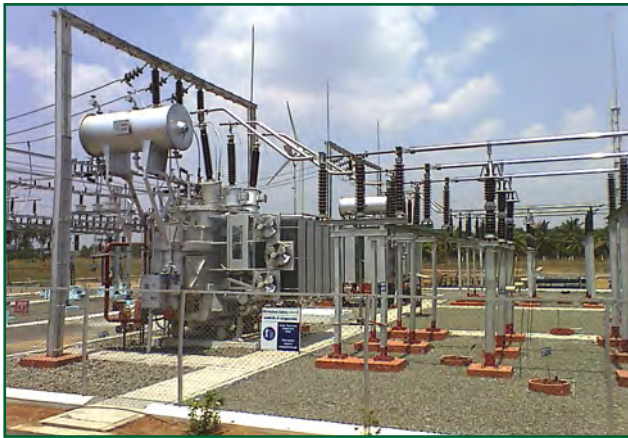
Peethampalli Substation where power quality measurements are underway
