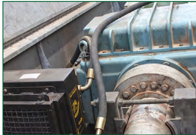
Gear Oil Cooler to reduce the Gear Oil Temperature
