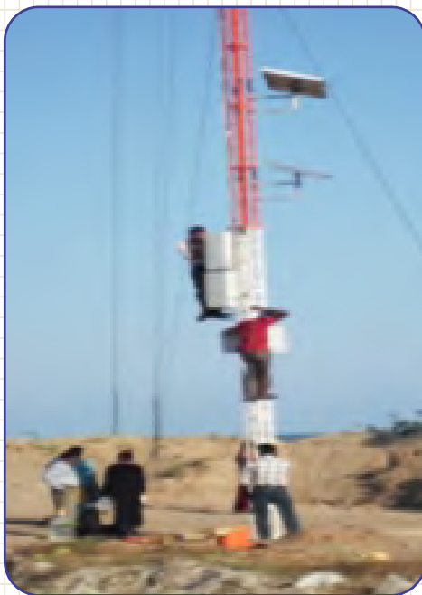
80m mast Ennore Port
