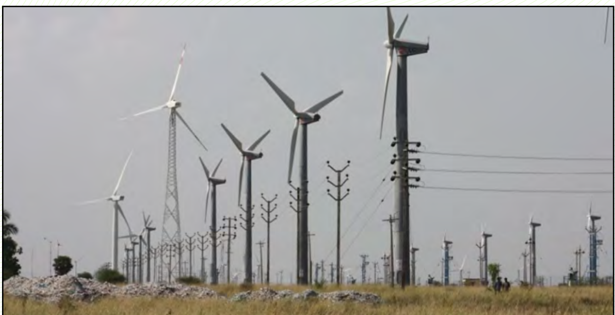
200 kW MICON Wind Electric Generators at WTRRS, Kayathar
