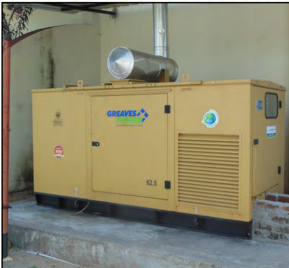
62.5 kVA Diesel Generator
