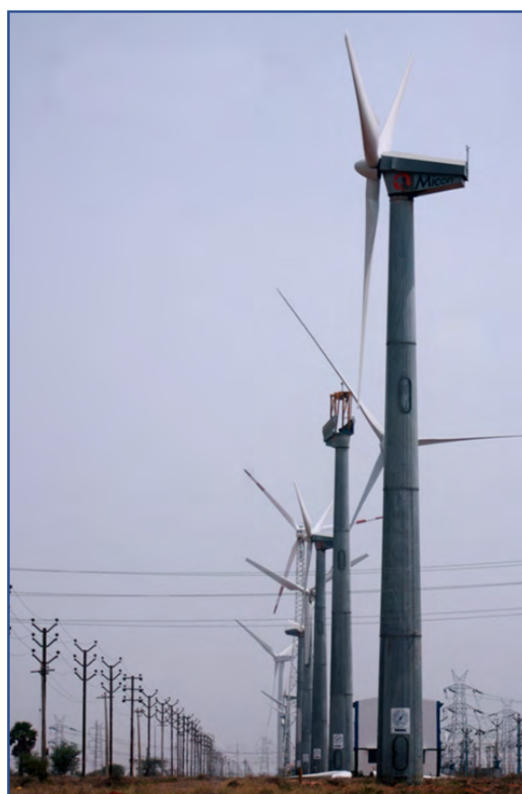
First Generation 200 kW MICON Wind Electric Generators
