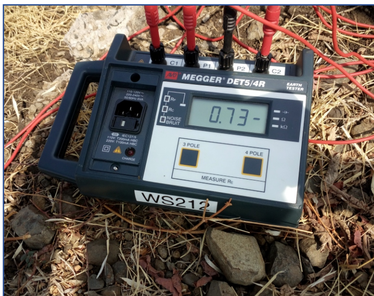
Earth Pit Resistance Measurement of 1000 kW WT at Richadewda, Ratlam District, Madhya Pradesh of M/s. XYRON TECHNOLOGIES LTD.
