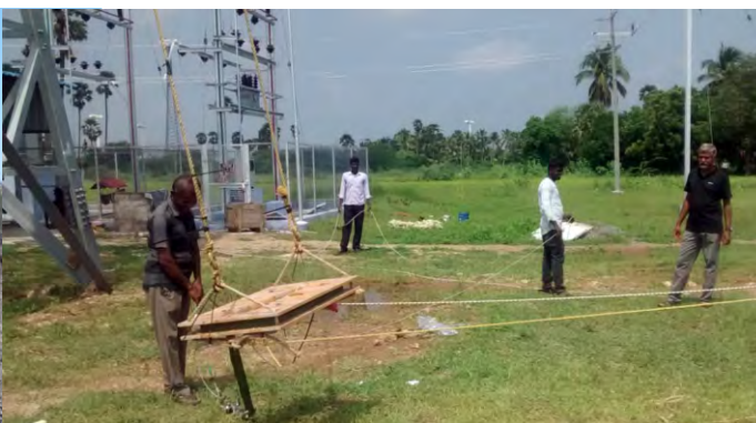
Para P57 Blade Load Calibration Test – Type Testing of Para 750 kW wind turbine of M/s. Para Enterprises Pvt Ltd
