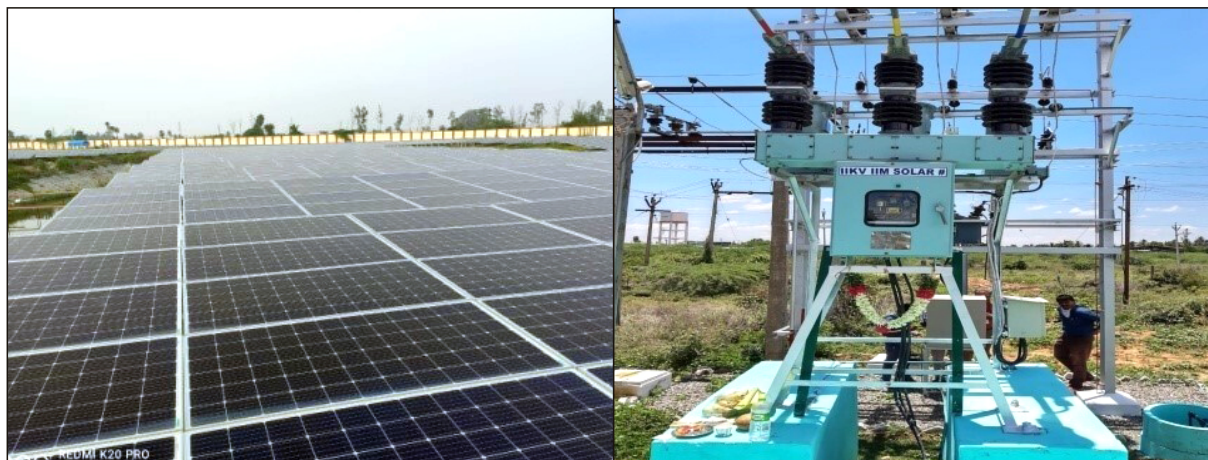
2 MW Solar Power Plant at IIM-Trichy Project Site Grid Synchronized from TNEB Sub Station
