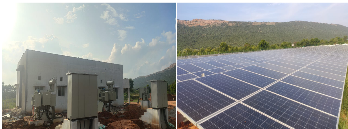
1 MW (AC) Ground Mounted Grid Connected Solar Power Plant at Madurai Kamaraj University (MKU), Madurai
