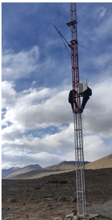
50 m wind monitoring station installed at Kargil
