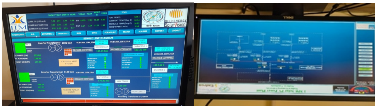
SCADA system data view
