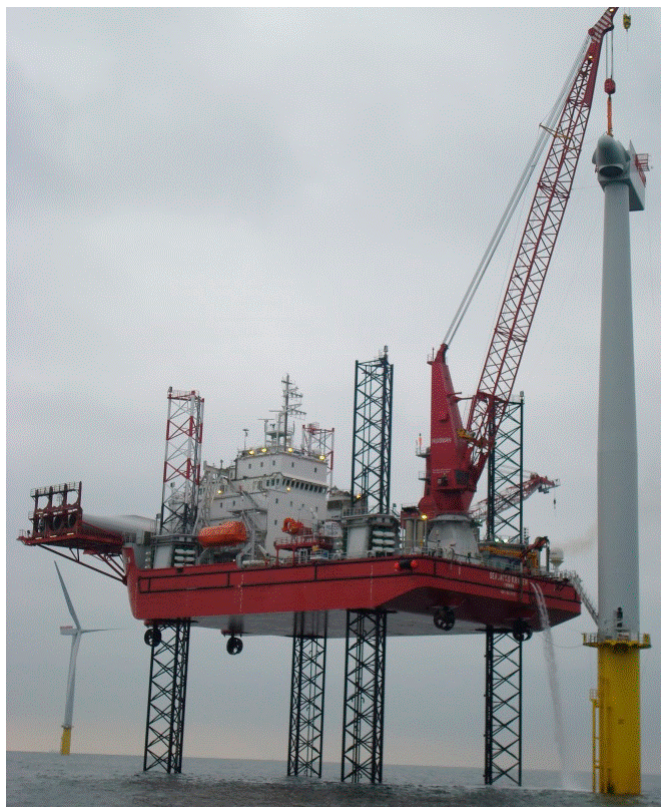
Figure 80 - Wind turbine installation vessels
