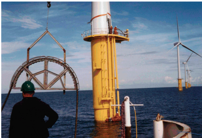
Figure 84 - Cable installation adjacent to a wind turbine
