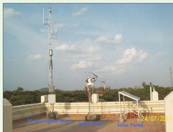
Fig 7: View of SRRA station at Vellore
