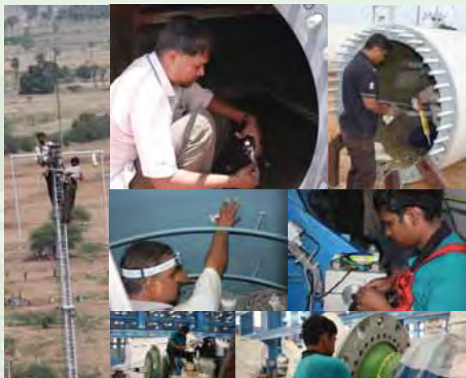
Elecon 600 kW Blade, Site & Factory Instrumentation
