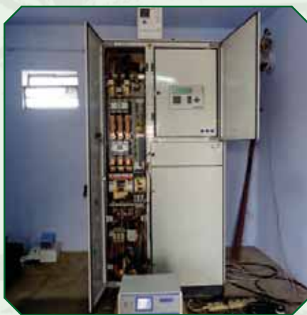
Power Quality Measurement in progress
