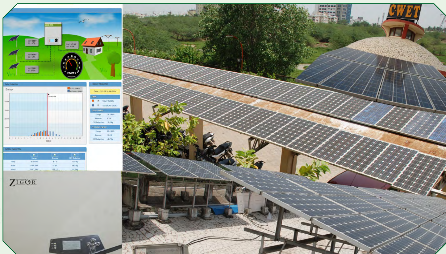
15 kW on grid SPV power project
