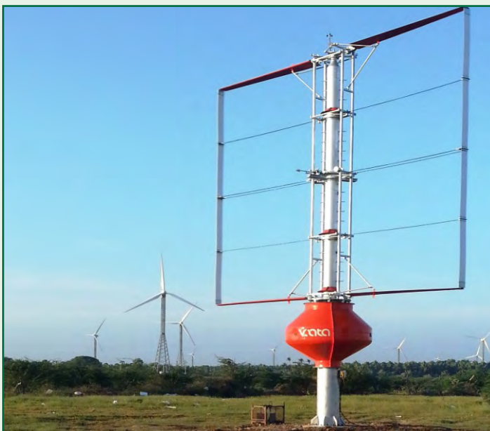
Typical view of 15 kW Vertical Axis grid-connected small wind turbine
