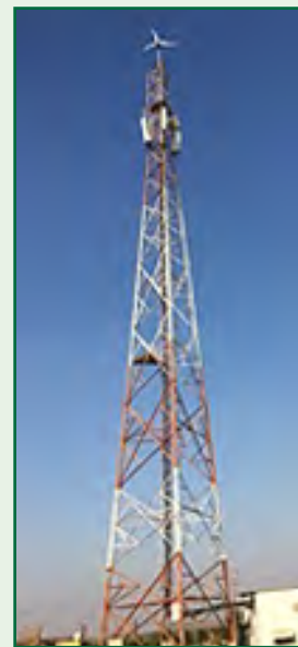
SWT installed on Telecom tower
