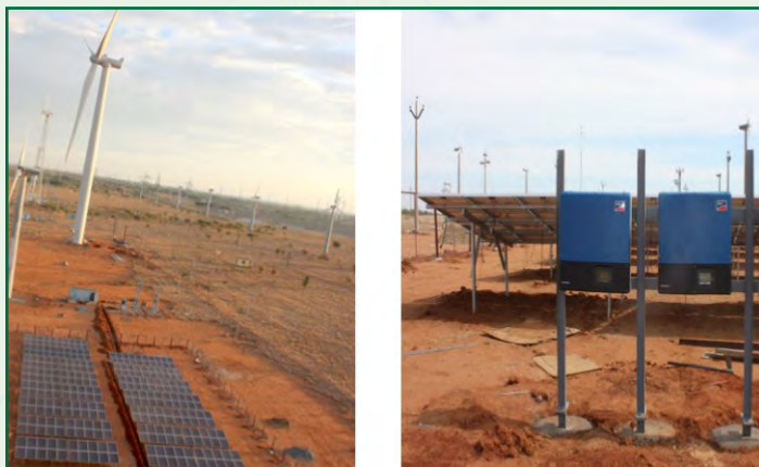
Grid Integration of 75 kWp SOLAR PV with 200 kW WEG @ WTRS Kayathar
