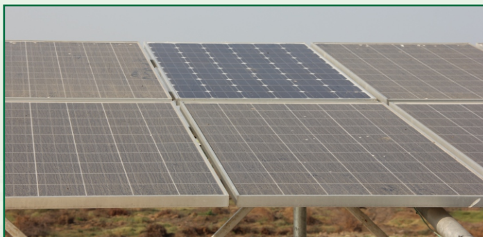
20 kW solar panels installed at rooftop after Vardah Cyclone & repair
