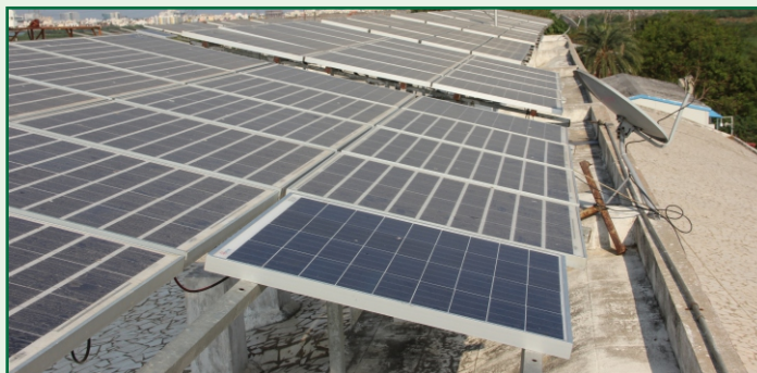
15 kW solar panels installed at rooftop after Vardah Cyclone & repair
