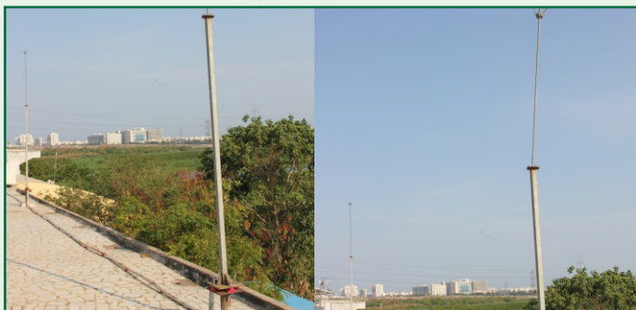
Lightning Arrester before & after Vardah Cyclone & repair
