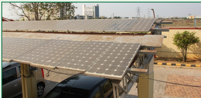
15 kW solar panels installed at car shed after Vardah Cyclone & repair
