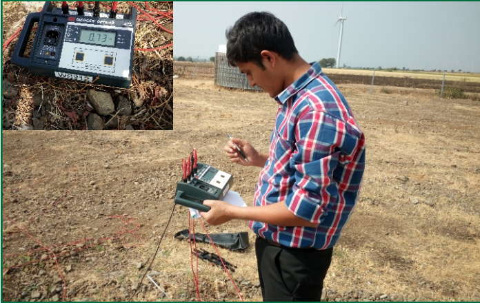
Earth Pit Resistance Measurement
