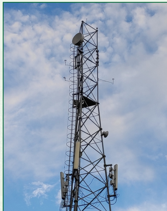
Image- Wind resource assessment sensors mounted on telecom tower
