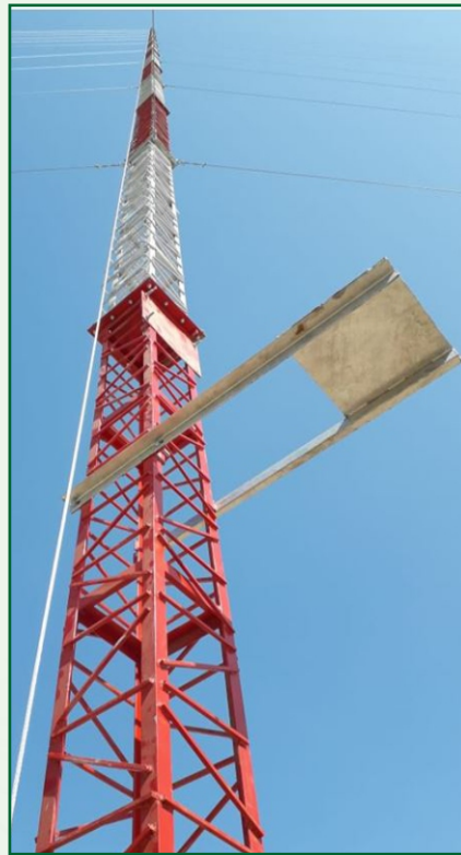
100 m integrated wind-solar mast installed at Gujarat
