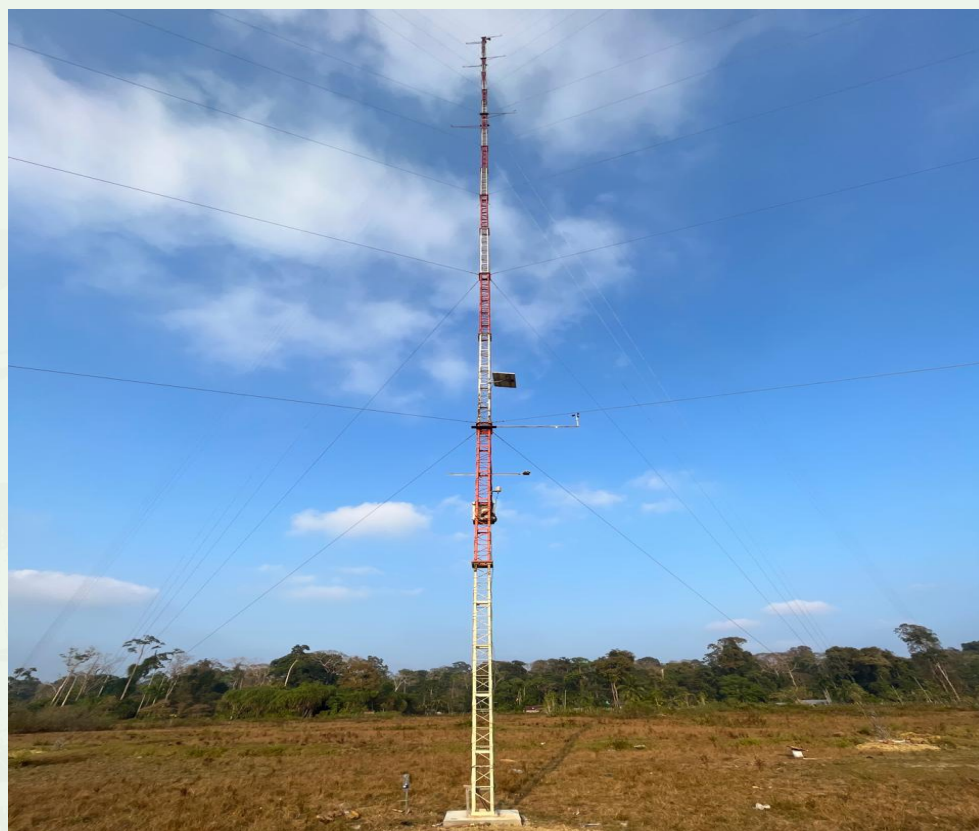
WMS Installed at Sigmundera
