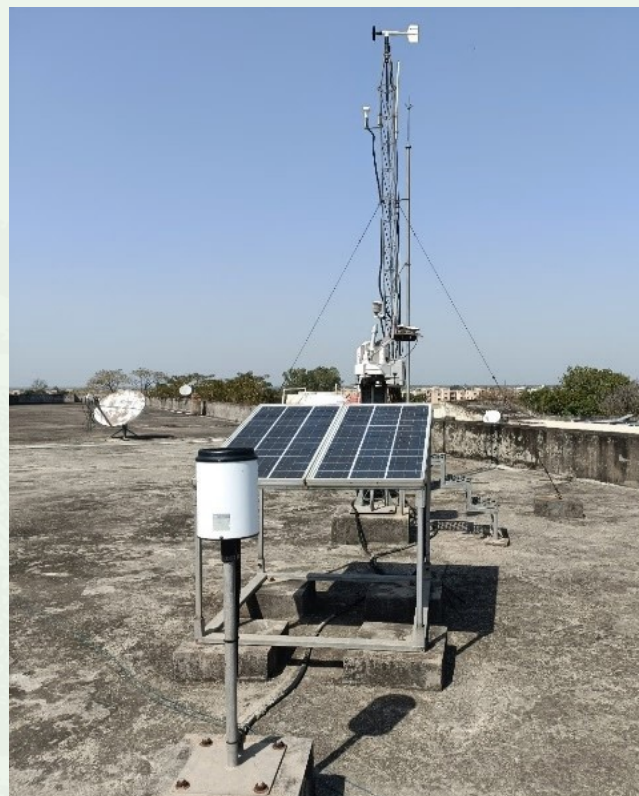
SRRA Station Installed in Madhya Pradesh
