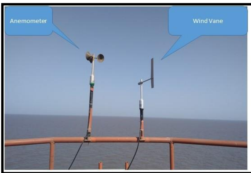
Figure 9: Anemometer and Wind vane setup Installed at the platform rail
